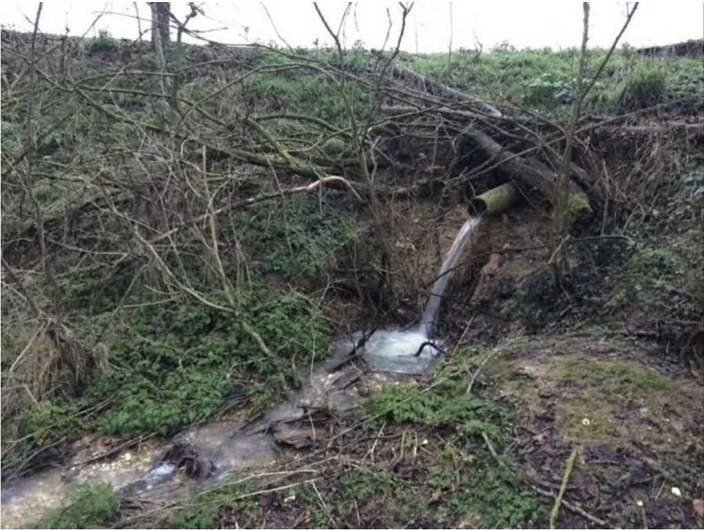
3. Land drain discharging into pit from substation site
