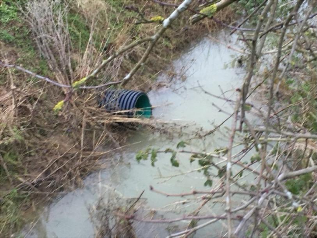
6. Land drain discharging into ditch near overhead cables, which feeds into Pit 2 near pylon adjacent to FP17 – 15 th January 2021
